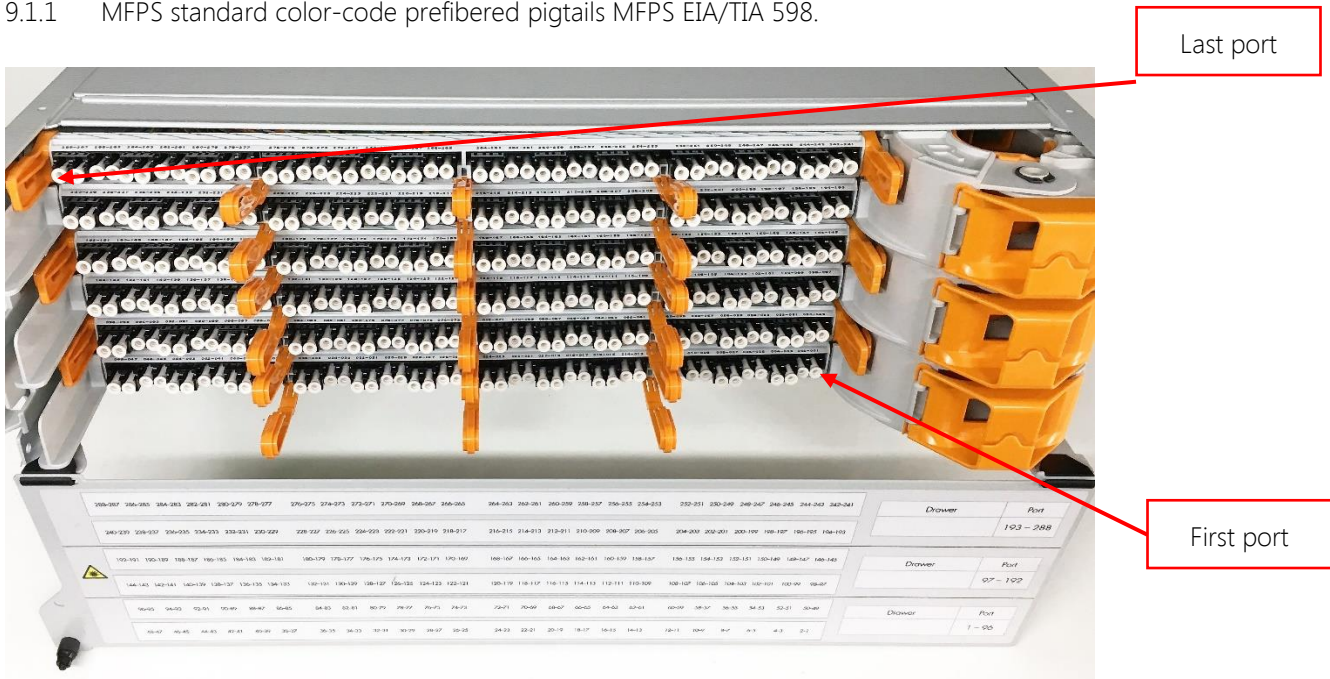
9.1.2 MFPS standard port numbering; starting from the hinge side, bottom is the first port (right side for a right orientated MFPS version, left side for a left orientated MFPS version). The opposite side on the top is the last port.
