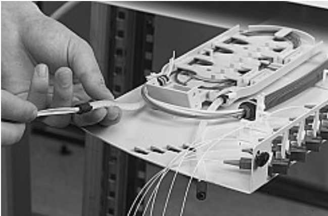
3.4.8 Feed the first 6 pigtails through the spiral tube and connect the pigtails.
