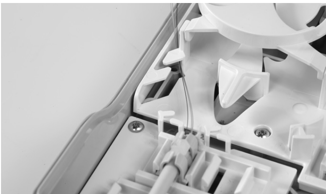
2.3.1 Route the fibers to the storage area. All fibers should enter through this port.
