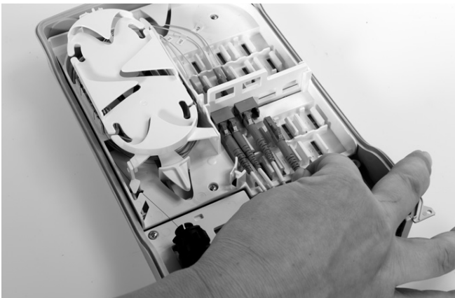
2.5.1 Install the patchcords into the designated adaptors.
