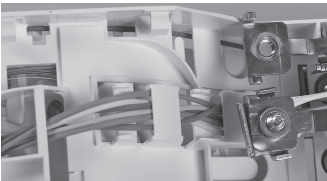
4.1.4 In order to have free fiber bundles at the organizer side the crossing of the bundles need to be shifted to the dedicated zone as shown.
