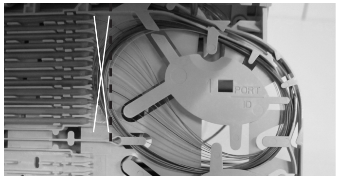
9.5.9. Wrong installation of loops around the island. Loops are passing the line and are too close to the splice holder.
